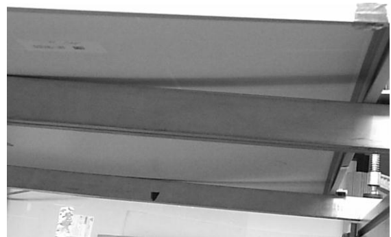
Fig.2, At a load higher than 2400 Pa the back sheet of module type #1 is pressed onto the supporting beam.
